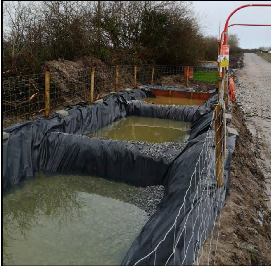
Figure 3-3 Multi-tiered settlement pond with stone filter
