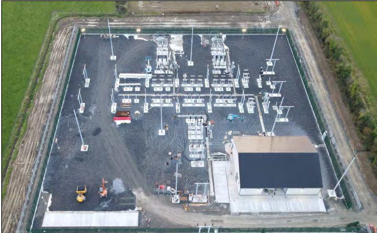
Figure 3.4: Example of a typical 110kV electricity Substation
