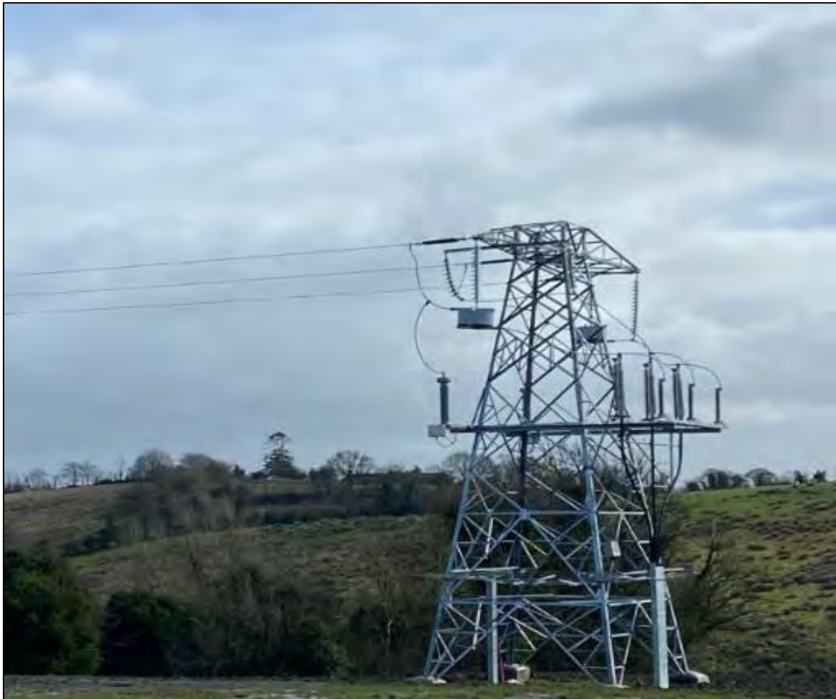
Figure 3.5: Typical Interface Mast
